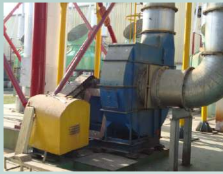
INDUCED DRAFT FAN
